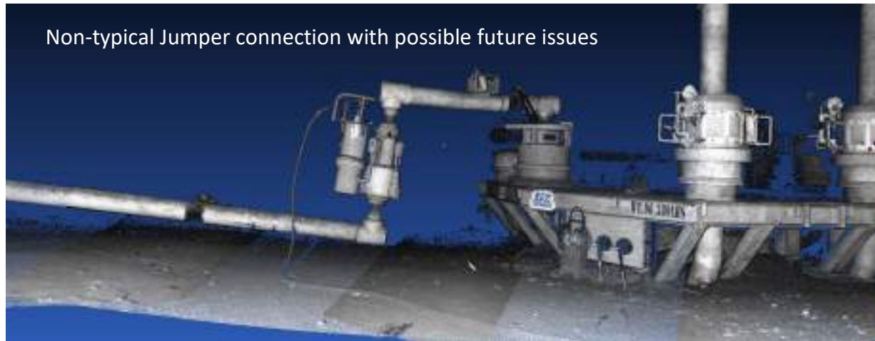
Typical jumper connection
